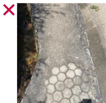
Too narrow and inconsistent paving
